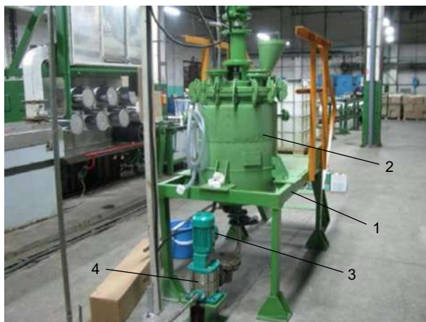
Fig. 2.16 Reactor: 1—platform; 2—vessel; 3—electric motor; and 4—hydraulic pump.
